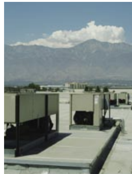
The outdoor condensing unit on the rooftop of the Cerenzia Foods warehouse.
